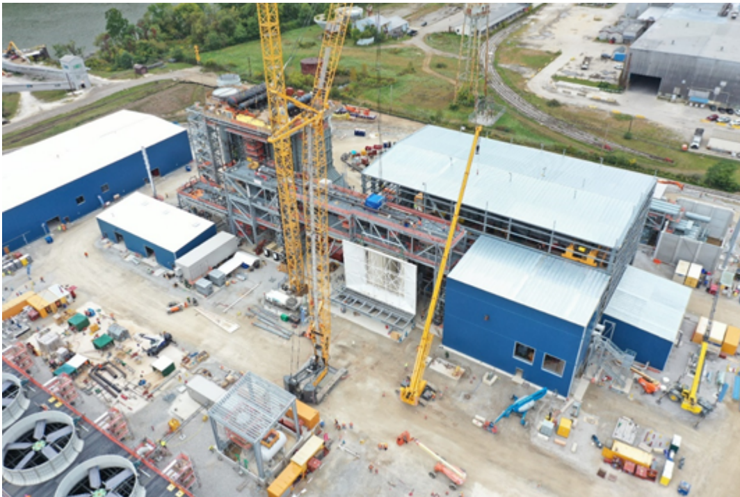
Long Ridge power plant under construction in Hannibal, Ohio. Photo courtesy of Kiewit.
