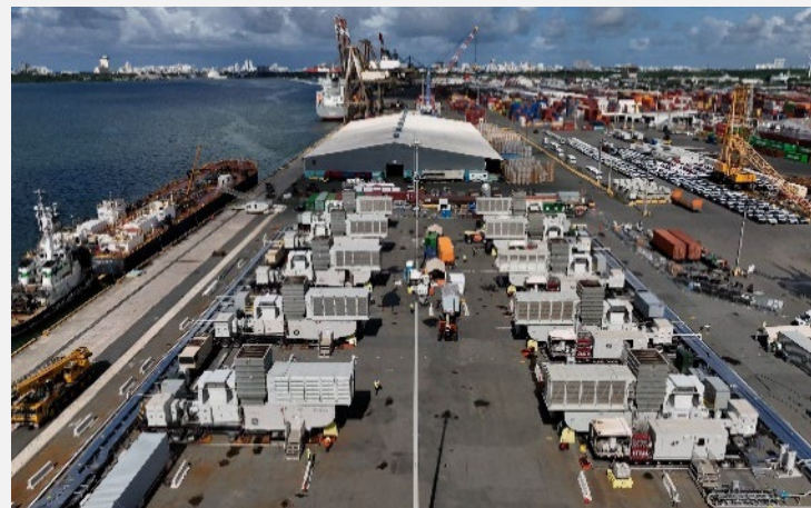
San Juan Fast Power 250MW
