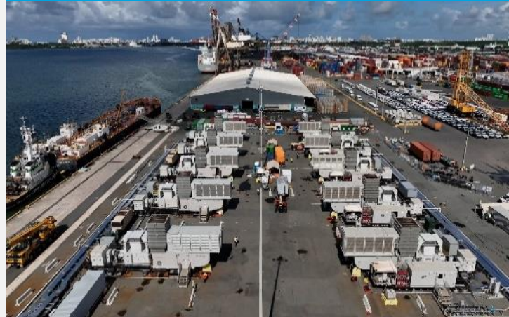
San Juan Fast Power 250 MW
